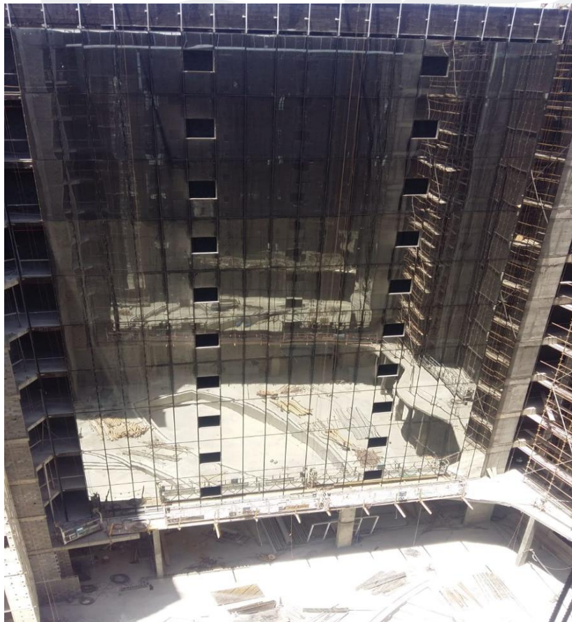
Installation of Aluminum Works (Brackets, Mullion, Rockwool, ACP Cladding and Glass and Application of Bitumen Paint)
