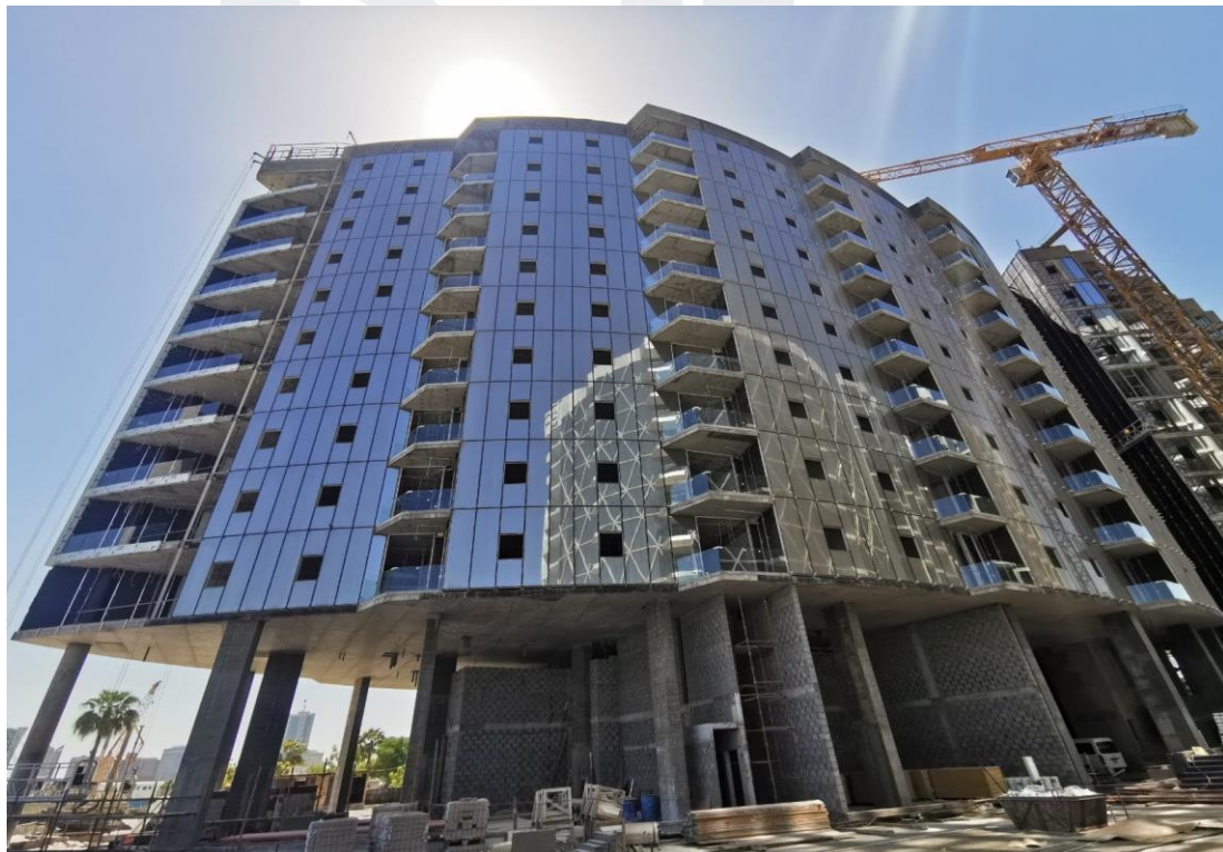
Installation of Aluminum Works (Brackets, Mullion, Rockwool ACP Cladding & Glass and Application of Bitumen Paint)
