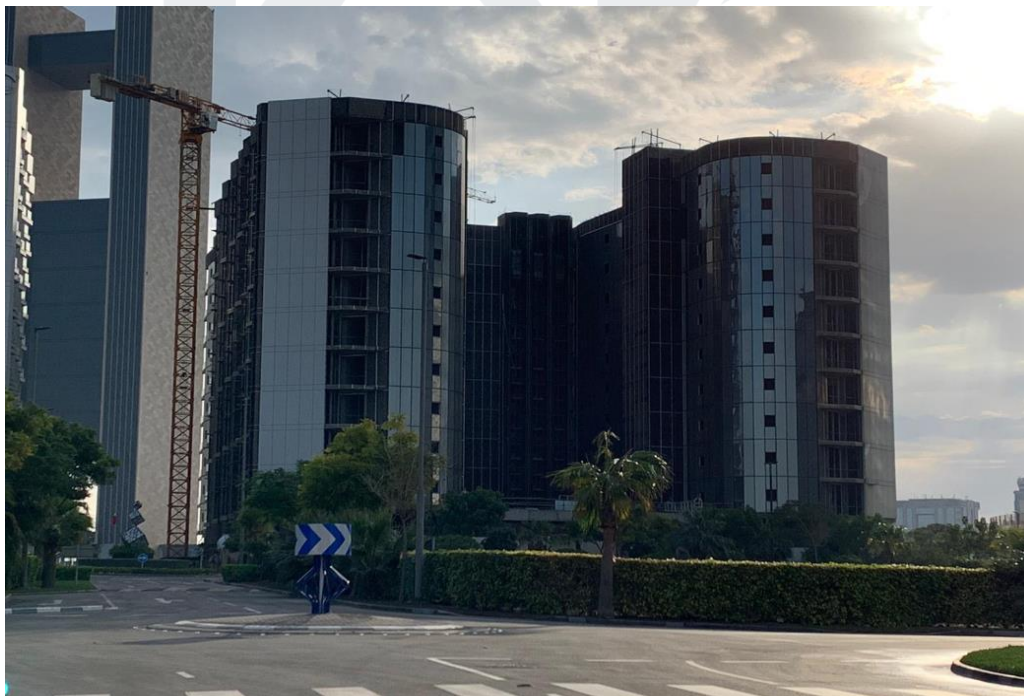
Installation of Aluminum Works (Brackets, Mullion, Rockwool ACP Cladding & Glass and Application of Bitumen Paint)
